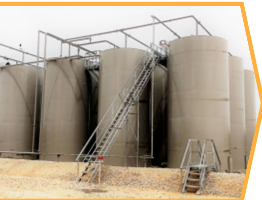
Impressive LLOX Algoa #1 & #2 Production Facilities
